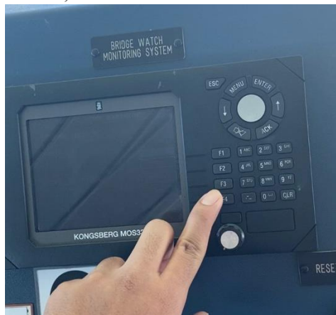
Figure 8. Bridge Watch Monitoring System
