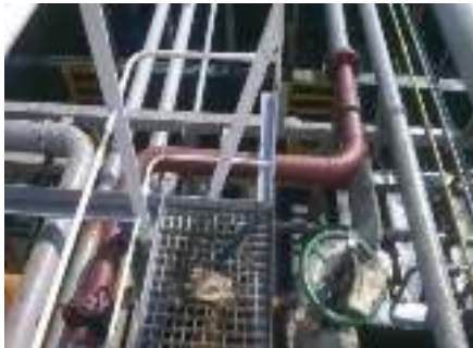
Gambar 8. Pipa Hidrolis Cargo Pump
