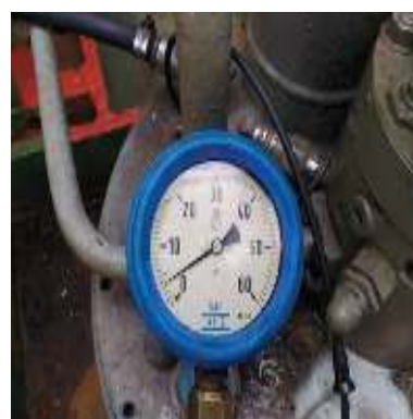
Gambar 9. Purging Cargo Pump pressure
